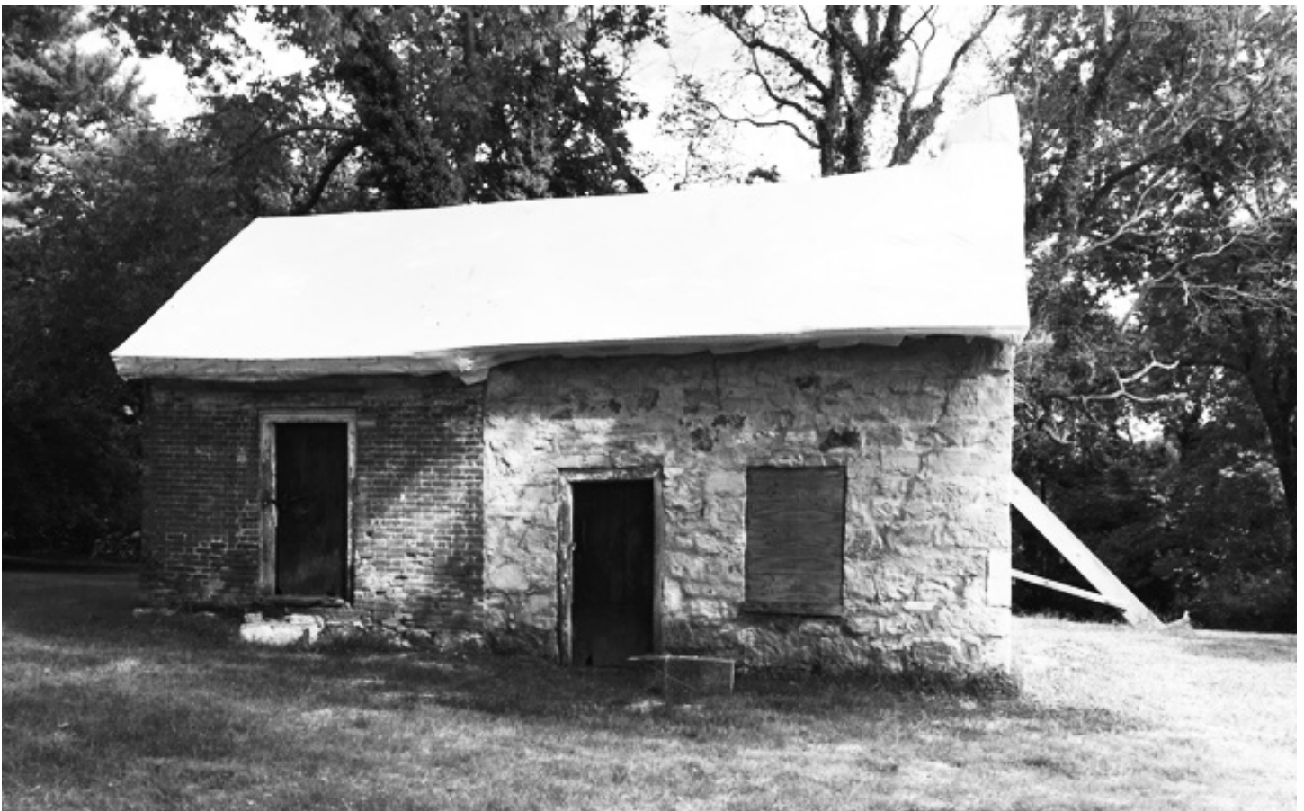
A new protective Shrink Wrap from Belfor, an international property restoration company, protects the roof of the smokehouse/kitchen
